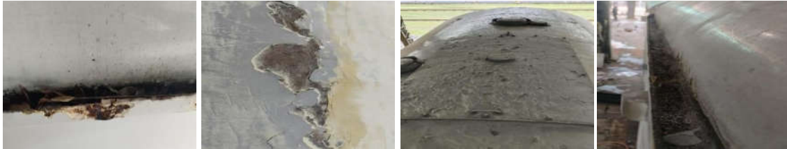
Fig. 1. Corrosion on Mild Steel Train Roofs
